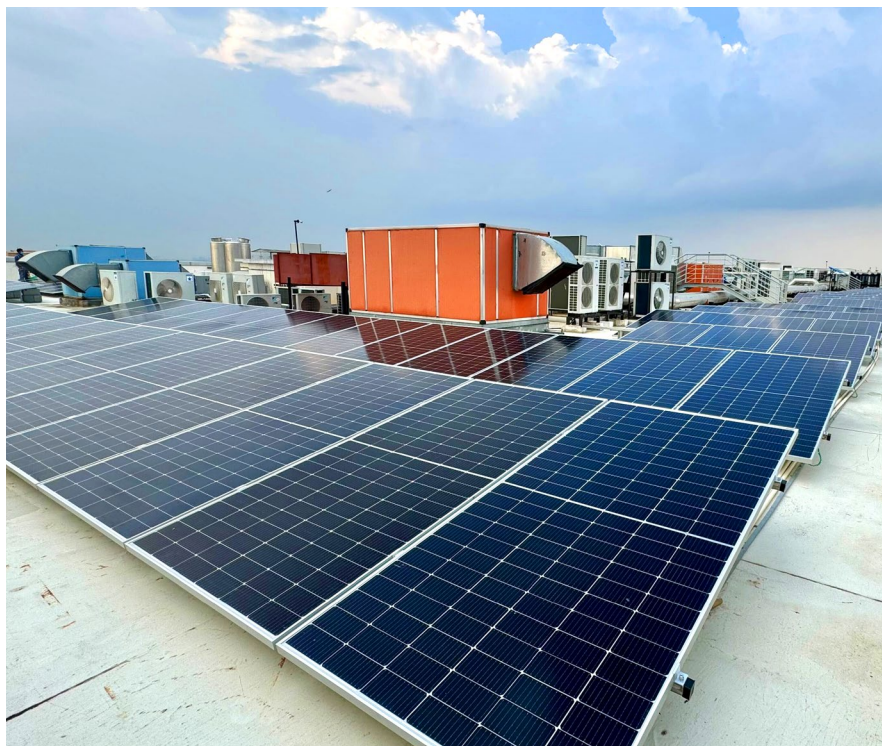
Solar panels on the rooftop of the Marvell site in Bangalore, India.
